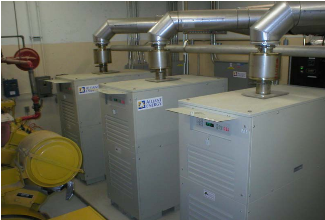
Figure 6-12 Capstone 30 kW Turbines Installed at the Albert Lea, Minnesota Wastewater Treatment Facility
