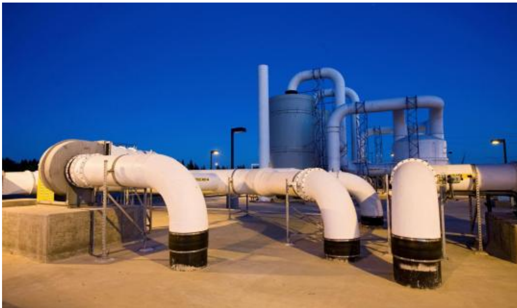
Figure 6-10 Example of a Typical Odor Control Installation at a Wastewater Treatment Plant
