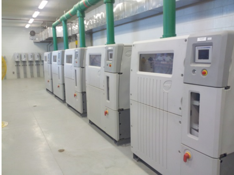
Figure 7-5 On-Site Chlorine Generators
