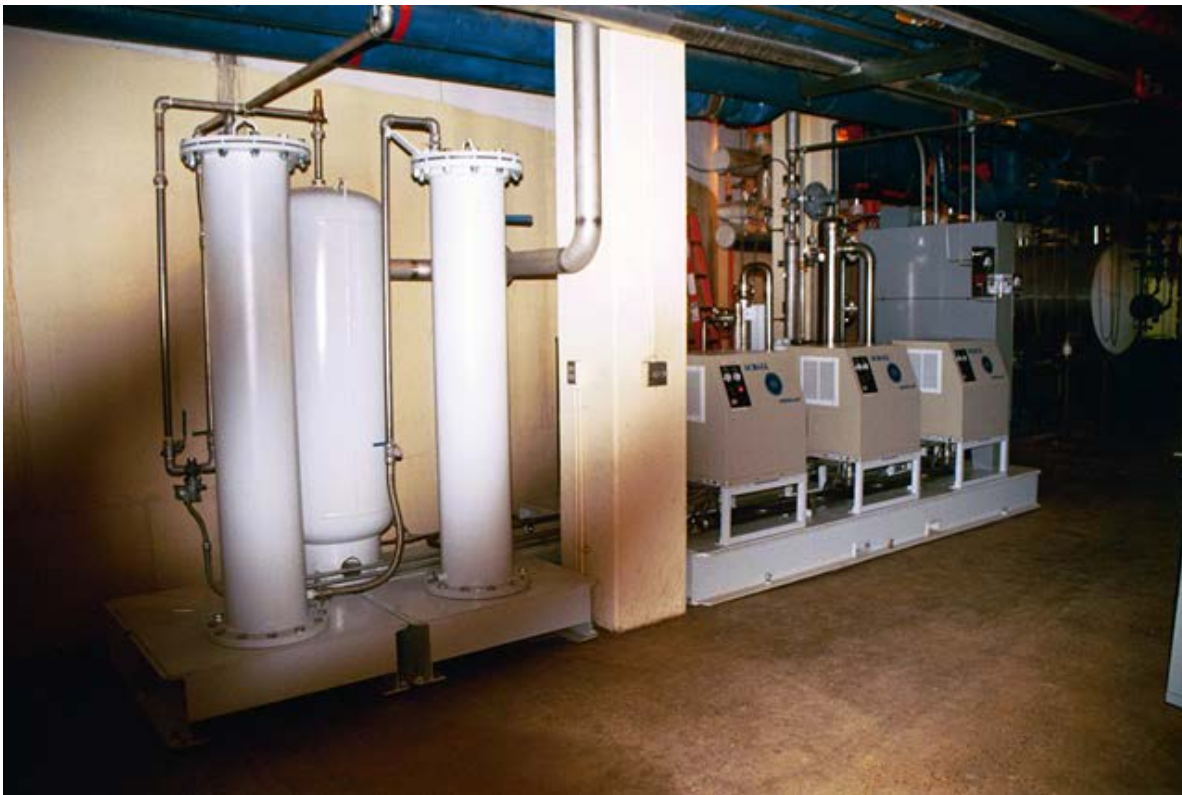
Figure 5-1 Biogas Cleaning System for CHP Installation at Albert Lea, MN WWTF
